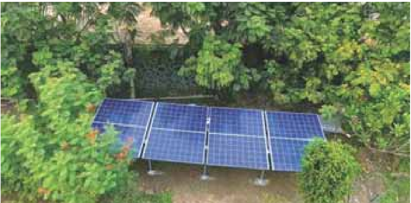
Renewable Energy initiatives undertaken at Blue Star's manufacturing facility
