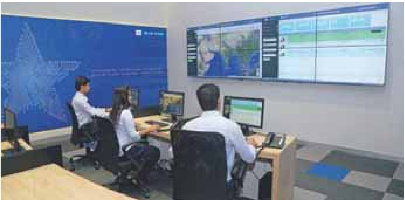
Remote Monitoring Services centre
