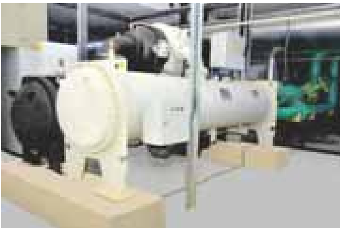
Installation of centrifugal and air cooled screw chillers, along with VRF V Plus system for Meenakshi Infrastructure, Hyderabad
